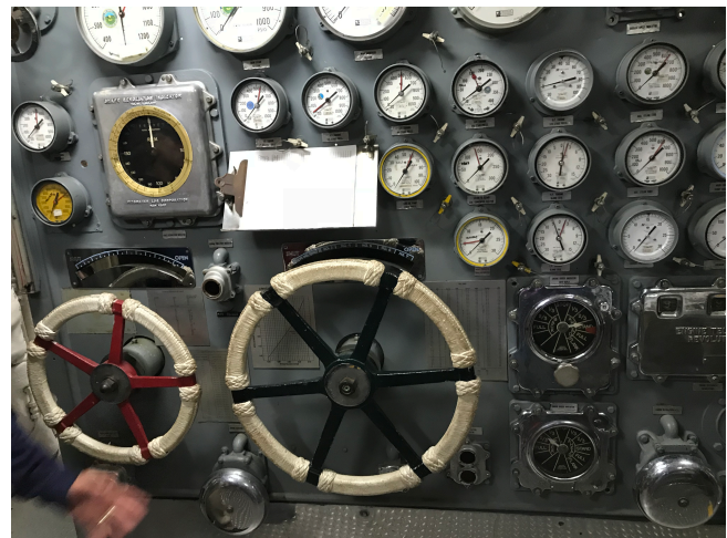
Figure 3, control valves for steam to a turbine.
