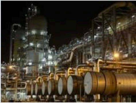
A Shell-owned ethylene cracker plant on Pulau Bukom,
